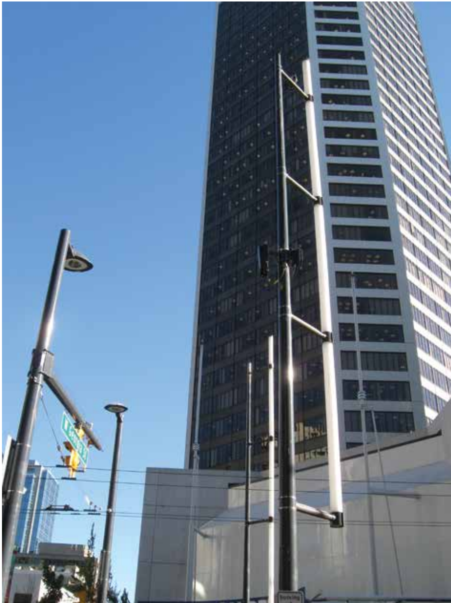
Small cell attachments to decorative street lights (the white vertical element is the light)
