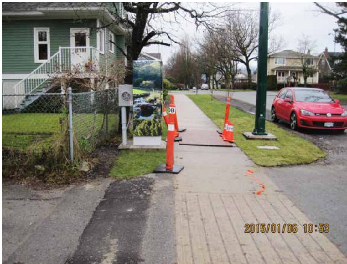
Close-up of connection cabinet
